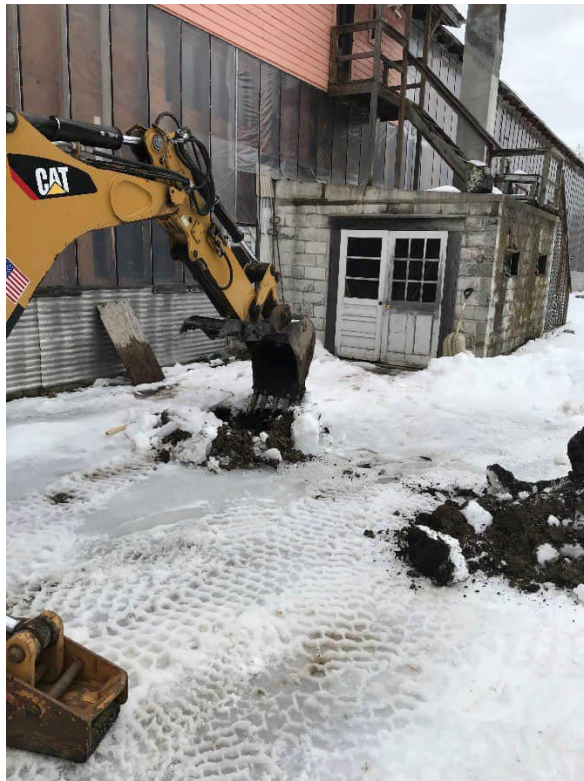
Photo #6: A view of Test Pit 1 (former UST location) on the southern side of the Recycling Barn facing east. Note: boiler located in cinder block room in background.
