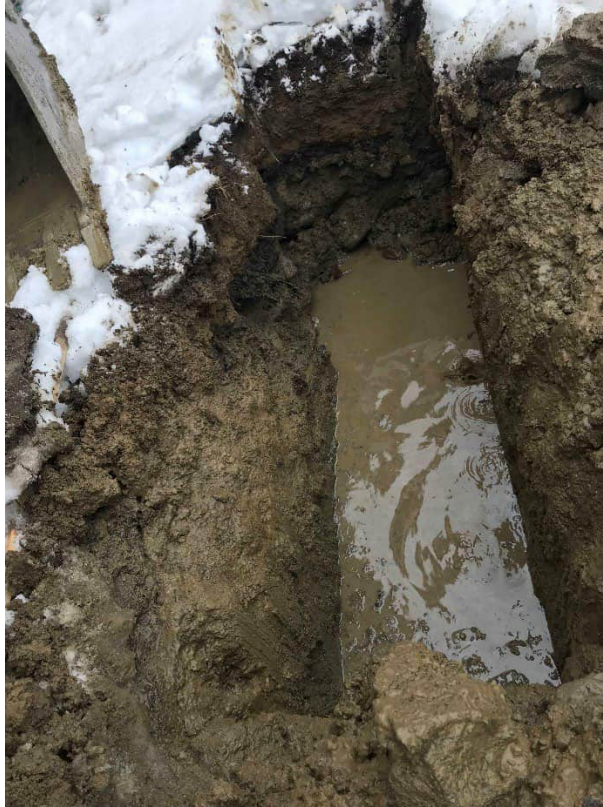
Photo #7: Another view of Test Pit 1, note: shallow water and floating sheen.
