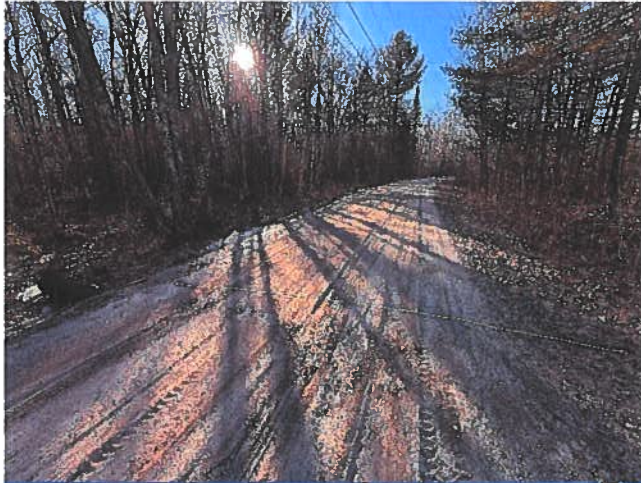
Figure 1: Culvert near 9 Birchwood Lane. Slight erosion visible on southern side of road. Traveled way appears to have shifted southward. This section of road is approximately 20 feet across.
