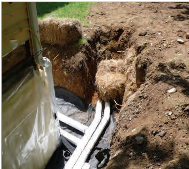
The Two Photographs Show The Town Office Energy Work: Excavation and Insulation of Foundation Walls. Photos: Chet Rice
