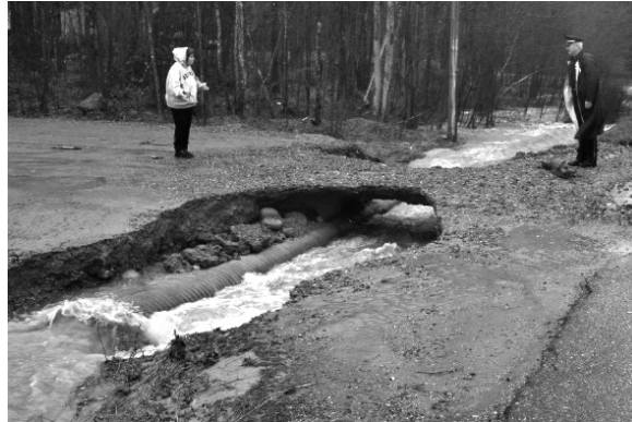
A road washout in Ellsworth, ME caused by a clogged culvert left residents stranded for several hours. Photo by Steve Fuller, 2015, The Ellsworth American
