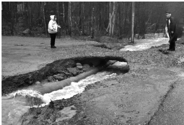
A road washout in Ellsworth, ME caused by a clogged culvert left residents stranded for several hours. Photo by Steve Fuller, 2015, The Ellsworth American
