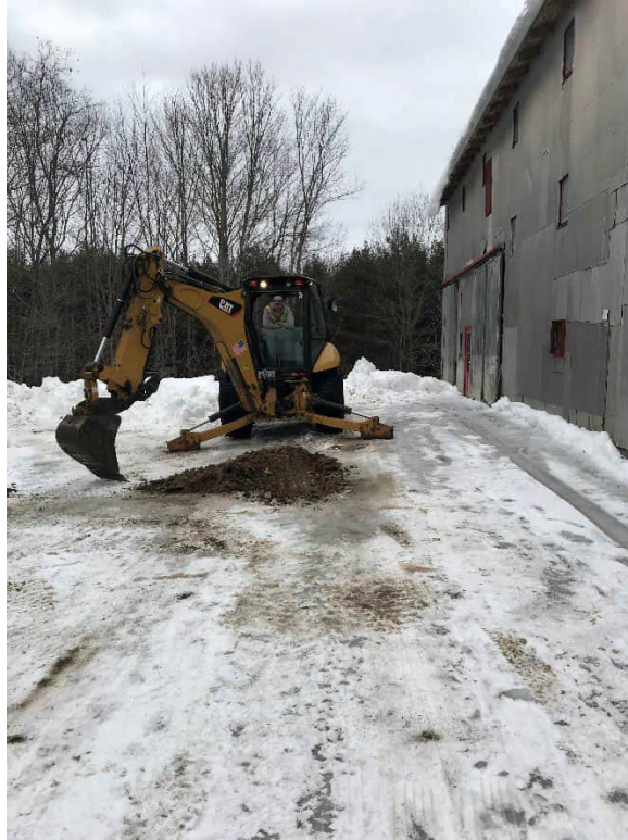
Photo #5: A view of Test Pit 4 in the “Antifreeze Pit” area of the site. Note: the machine was not able to break through densely packed and frozen material to examine this area and collect a sample.
