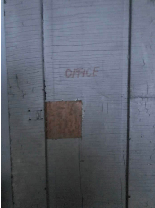
Photo #13: A view of paint sample collection location on painted office door near first floor boiler room. Note: paint removed down to bare substrate (wood) for sampling.
