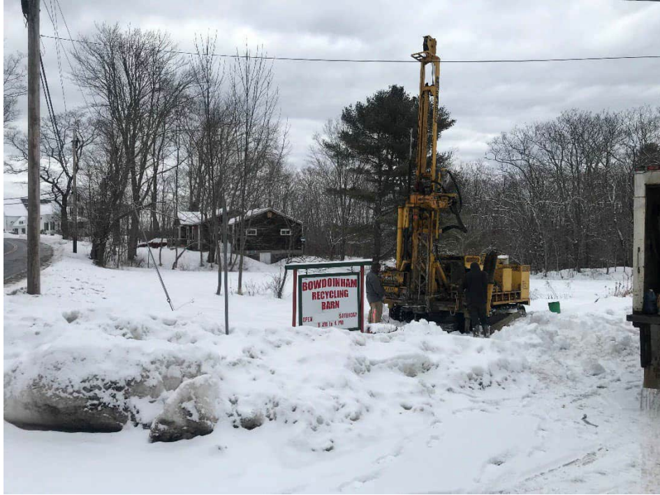
Photo #1: A view of drillers installing upgradient monitoring well along Post Road facing north.
