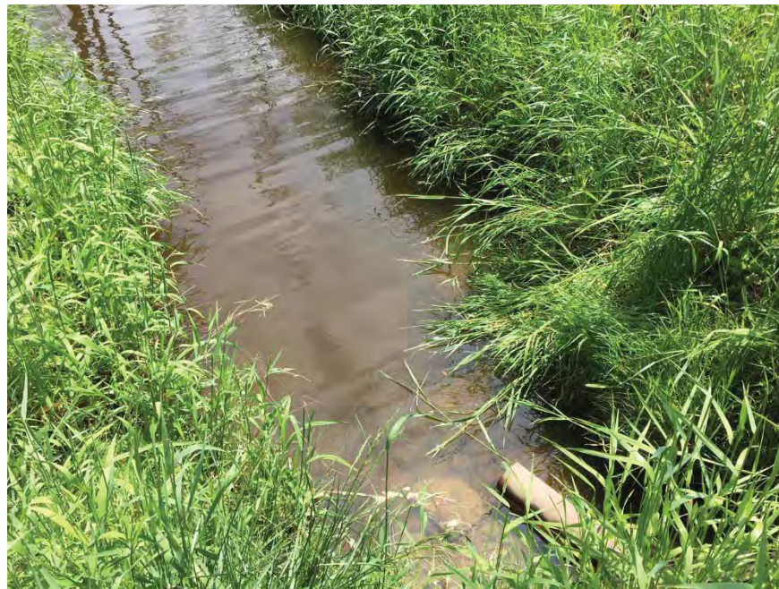
Photo 19. Small metal pipe draining into the trench/Cathance River. Stantec. June 14, 2019.
