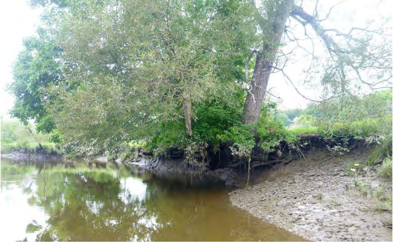
Looking south from River Road bridge area towards proposed vegetated retaining wall stabilization area. Low Tide 9:47am [Photo Time – Date: 8:10am – 8/13/18; Flow Tide]
