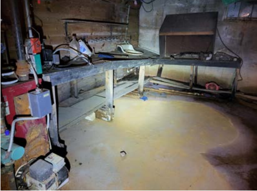
Degraded shelving unit and wall system
