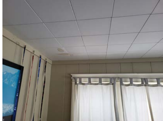
Water stained ceiling tiles
