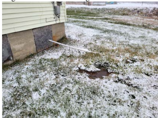
Saturated soils on rear of Building
