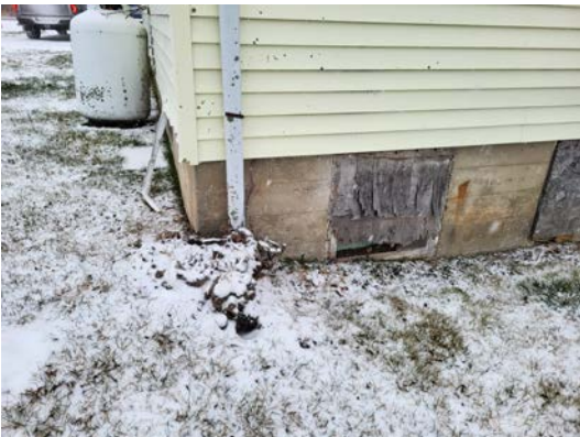
Downspouts appear to deposit water along foundation
