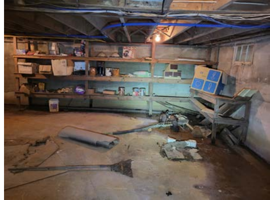
Shelving system is rotten
