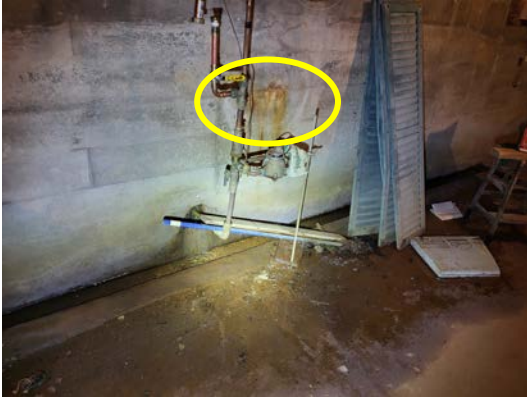
Water pouring in foundation wall
