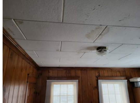
Water stained ceiling tiles
