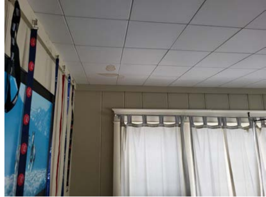
Water stained ceiling tiles
