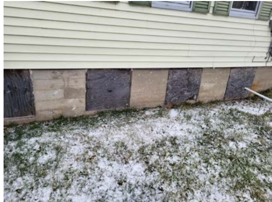
Degraded window coverings on foundation
