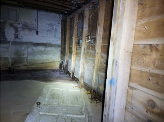
Pooling water and degraded wall system
