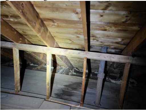
Signs of water impact round this plumbing vent stack
