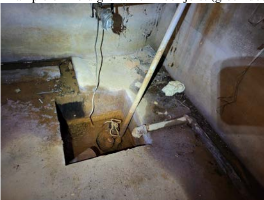
There is a sump pump
