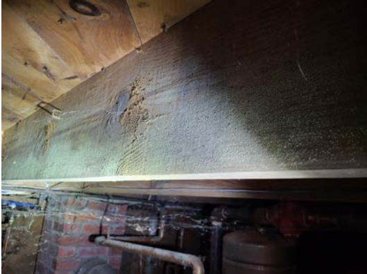
Example of mold growth on floor joist (green dots)
