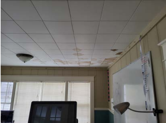
Water stained ceiling tiles
