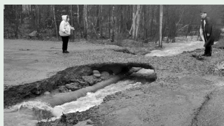
A road washout in Ellsworth, ME caused by a clogged culvert left residents stranded for several hours. (Photo by Steve Fuller, 2015, The Ellsworth American)
