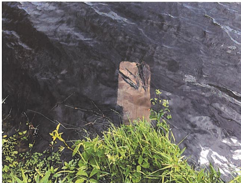
Photo 17. Exposed end of timber cribbing extending from shoreline, just south of wetland W-01TTA. Stantec. June 14, 2019.
